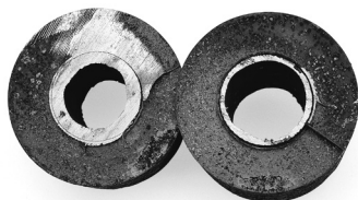
The cross section of the coil on the right shows how internal corrosion caused by improper piping, trapping and venting may destroy coils from the inside out.
